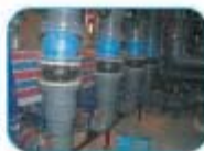
宁波东钱湖电化 Ningbo Dongqianhu Electrochemical
