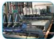
宁波核电站 Ningbo Nuclear Power Plant
