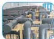
浙能东港电厂 Zhejiang Power Plant
